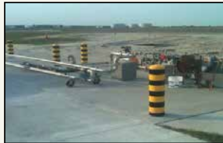
NS Mayport Helicopter Direct Fueling System
